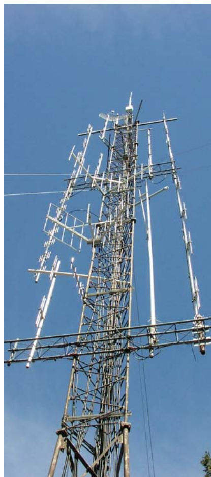
Top of the repeater tower.
